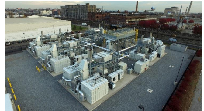
14.9 MW Bridgeport, Ct (FuelCell Energy)
